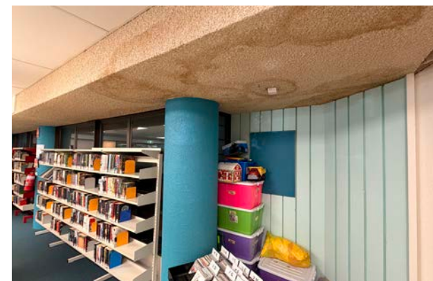
Water damage to ceiling
